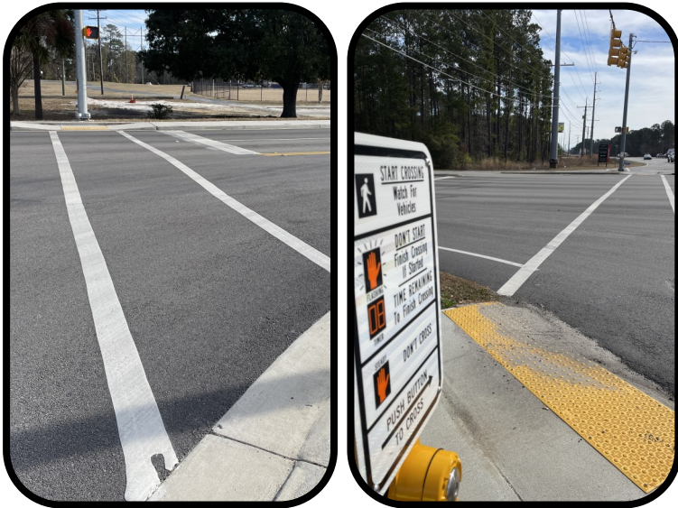
New pedestrian accommodations are incorporated into planned construction projects, like at these intersections in Berkeley & Dorchester Counties.
