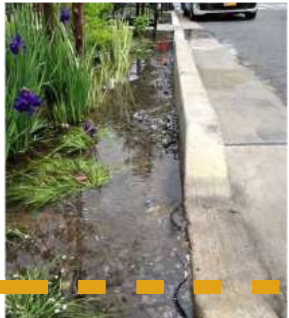
right: Bioretention within the right-of-way
