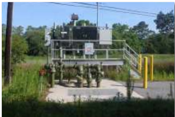
Charleston Water Systems Station (Source: BCDCOG Staff)
